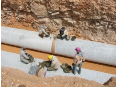
The pipes are coated with a protective layer before they are buried underground.
