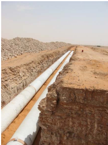
The transmission pipelines extend altogether for a length of 170 kilometers.
